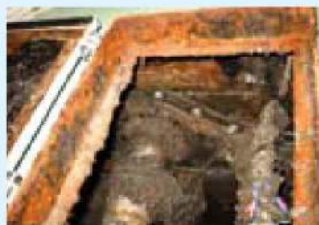
Conveyor for Raw Garbage
