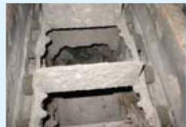
Fly Ash Conveyor: Dust Conveyor Under Boiler
