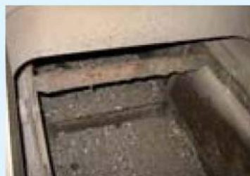
Fly Ash Conveyor: Dust Conveyor Under Boiler
